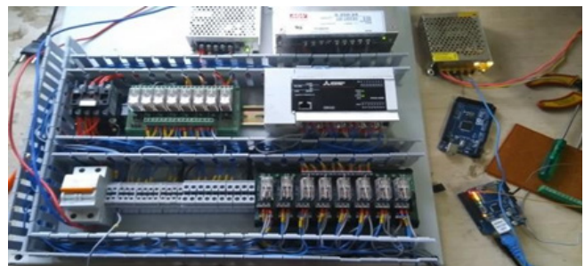
Figure 7: Wiring of Control Panel of Proposed machine
